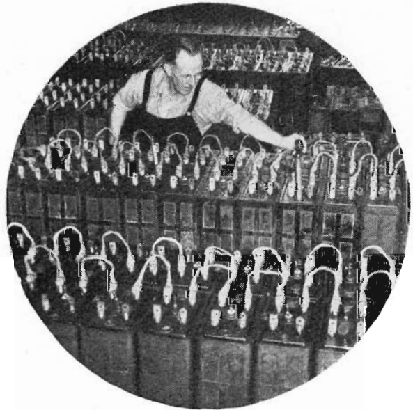
Battery charging is big business.
